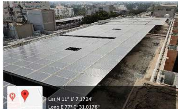
Solar Grid on Rooftop of Campus Buildings
