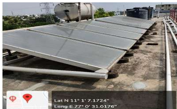
Solar Water Heaters of Rooftop
